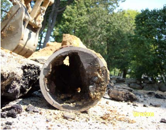
Tuberculated Old Water Main
