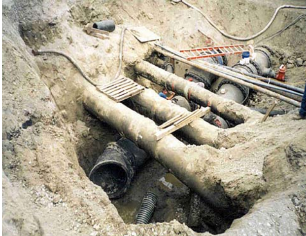
Twin 24-inch Connections
