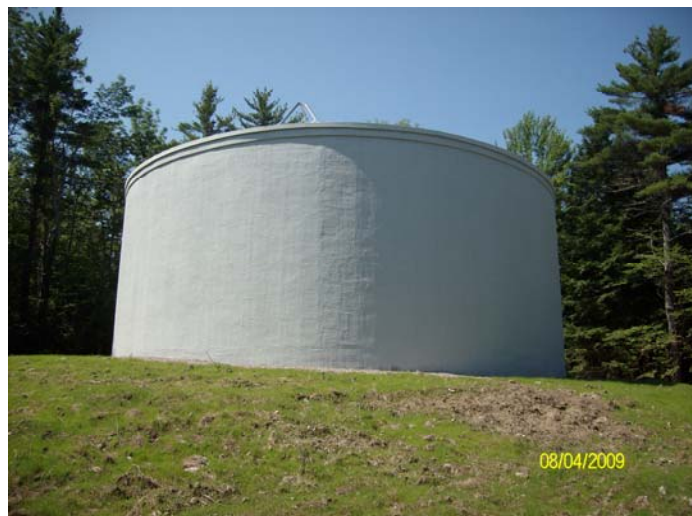
New Concrete Storage Tank in Place (existing tank is to the left)
