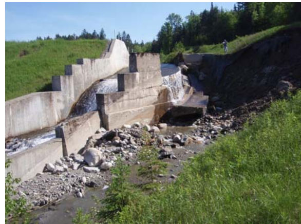
Damaged Lower Orange Reservoir spillway
