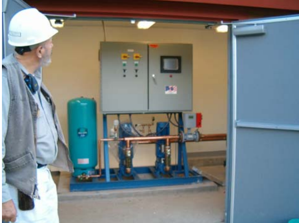
Packaged Pump Skid
