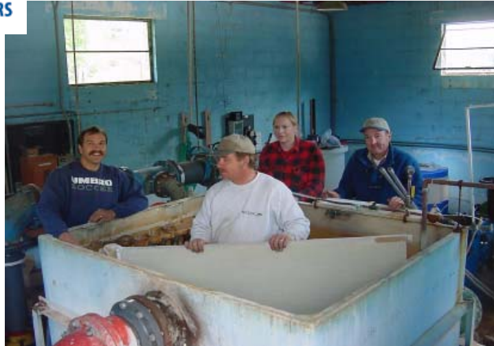
Andy Bladyka, Springfield Recreation Director and Harry Henderson, Director of Public Works observe installation of new equipment.
