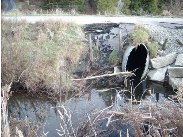
Metal arch structure damaged during Tropical Storm Irene
