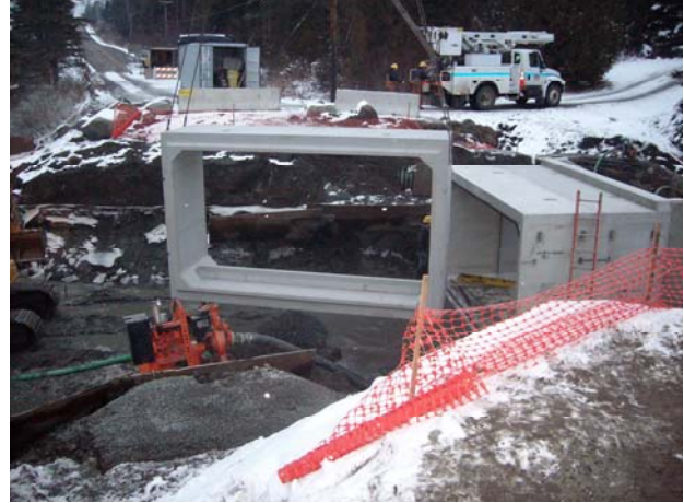
Construction workers set new 9 foot x 15 foot box structure (note baffler designed to hold natural stream material)
