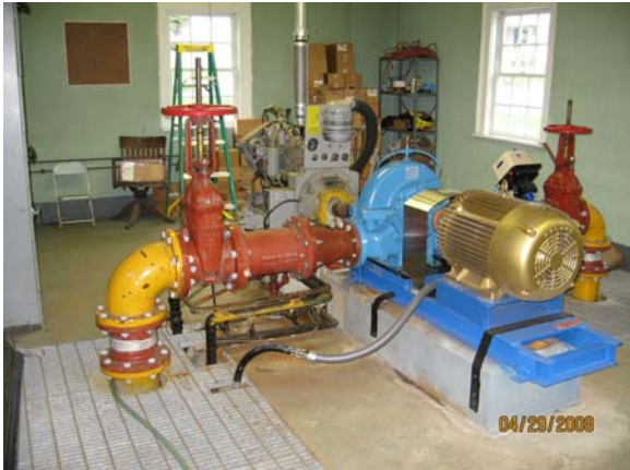
Original 50 hp pump #1
