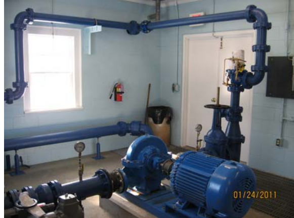
Replacement 75 hp pump #2
