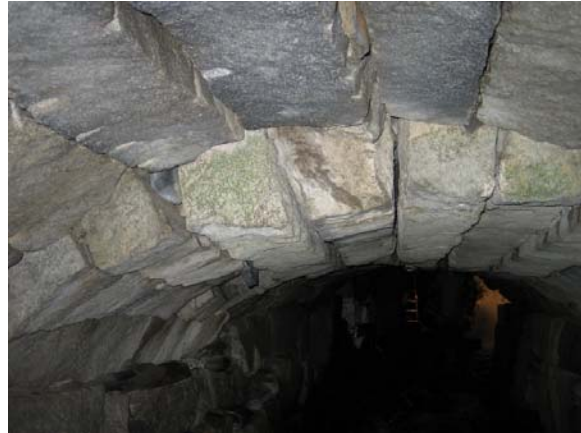
Failing Arch Culvert
