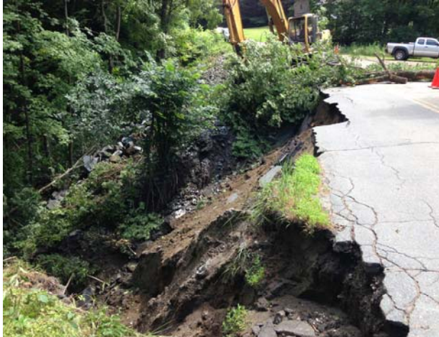
Slope failure after storm event
