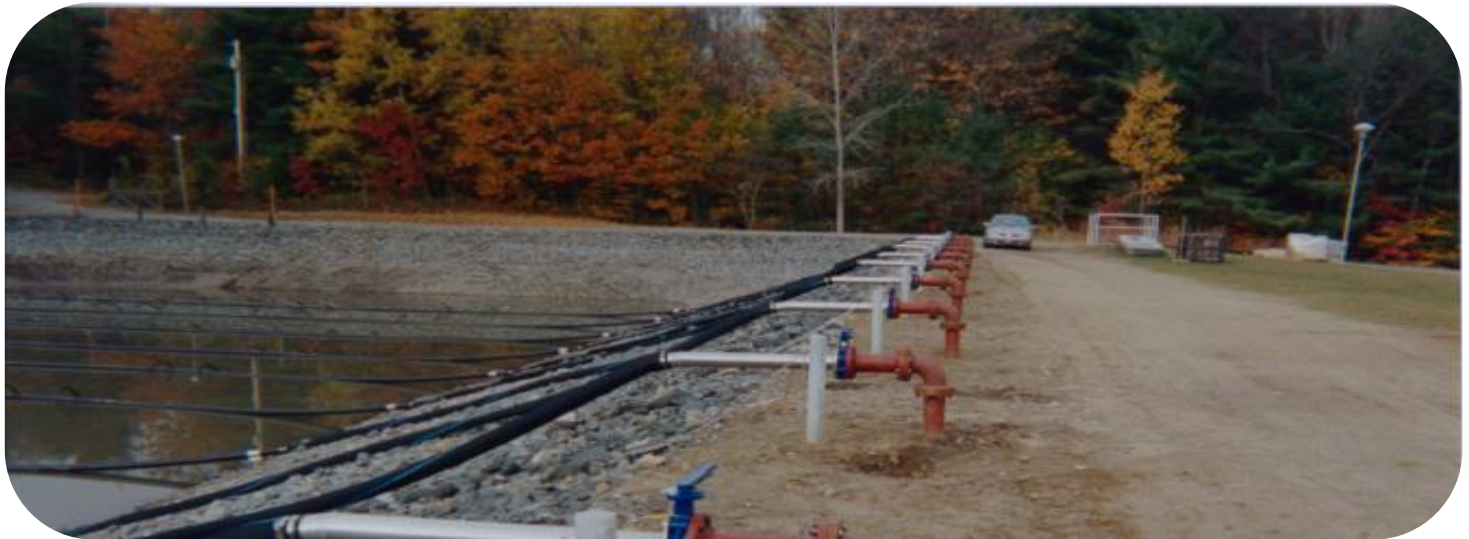
Lagoon Aeration System
