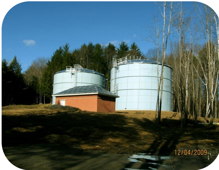
Completed Pump Station & Storage Tanks
