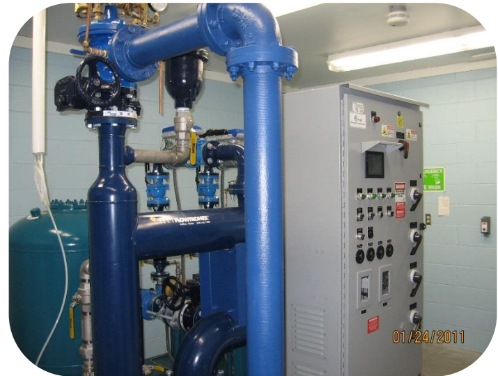
Pump Station Interior
