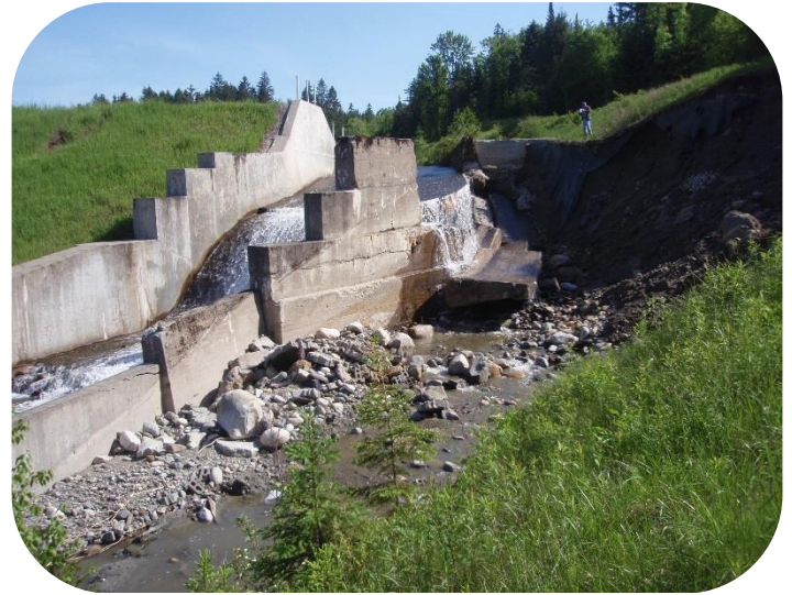
Damaged Lower Orange Reservoir spillway
