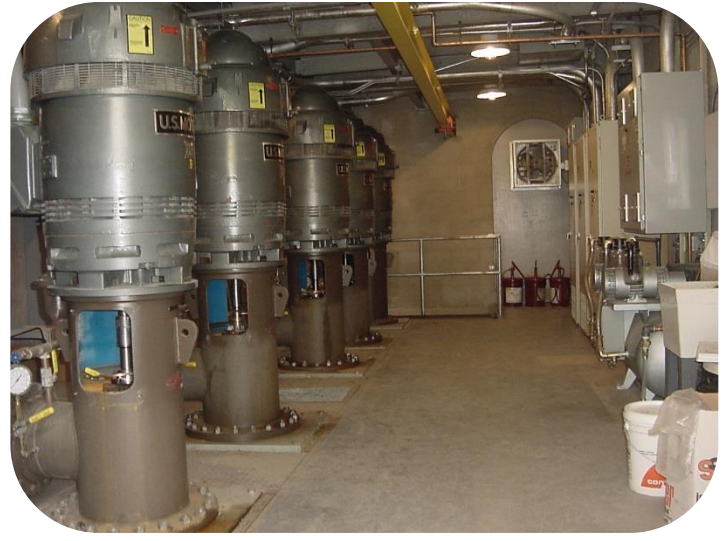
Raw Water Pump Station
