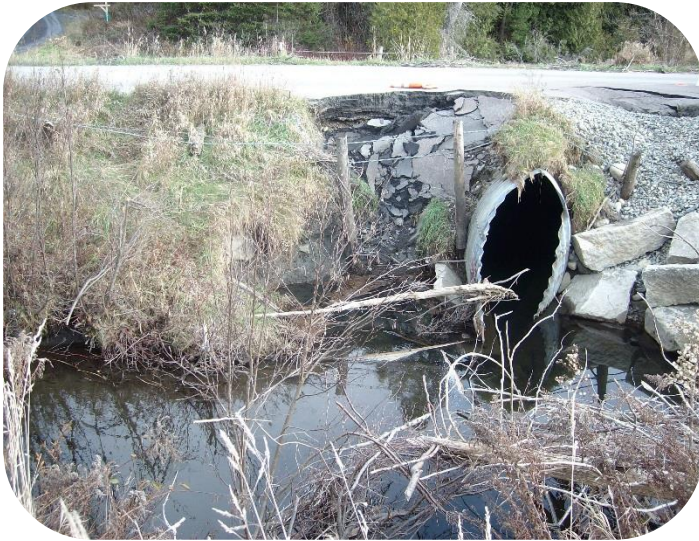
Metal Arch Structure Damaged during Tropical Storm Irene
