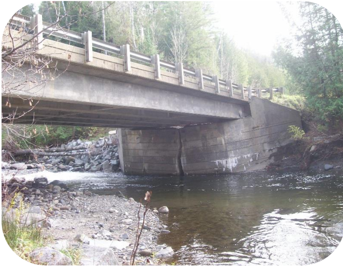
Damaged Structure, Note Abutment in River
