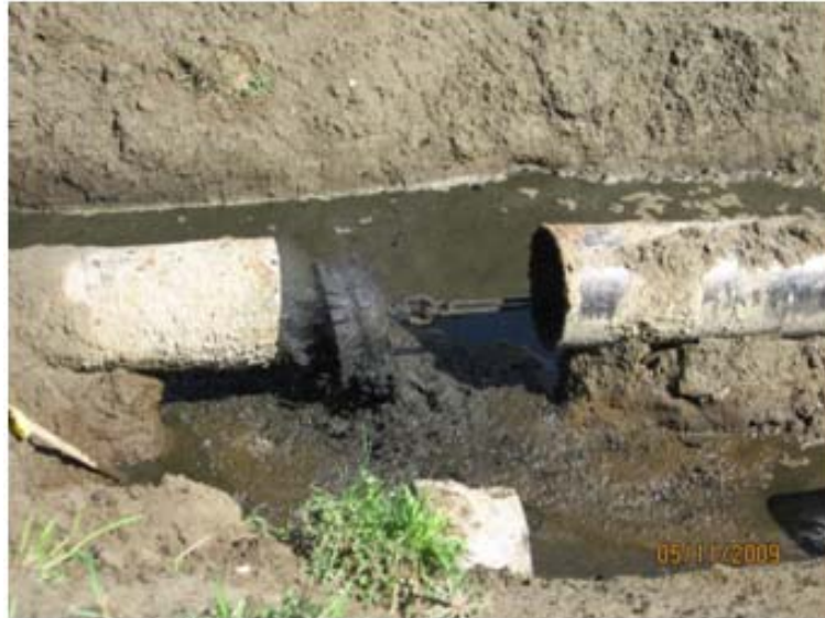
Cleaning scrapers are pulled through the water main to remove any mineral buildup that is present.
