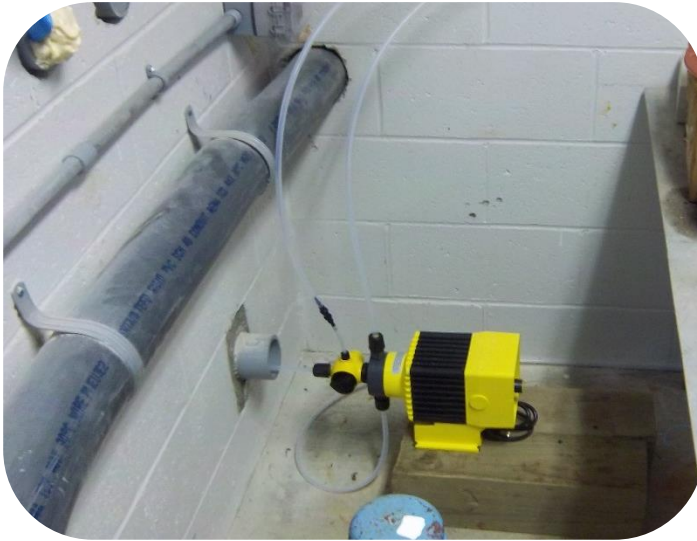
Chemical Feed Pump
