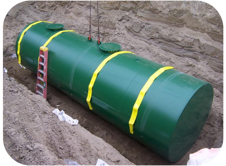
Stormwater Treatment Tank
