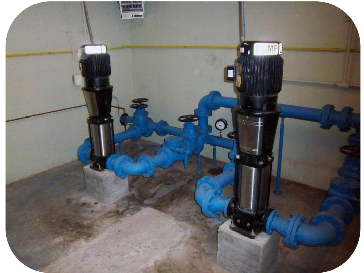
Raw Water Pumps
