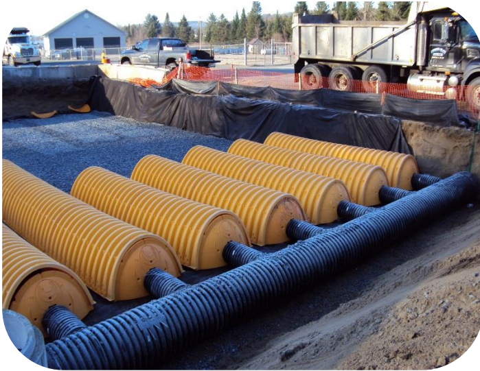
Manifold for infiltration system
